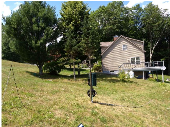
The control box under the antenna feed lines.
