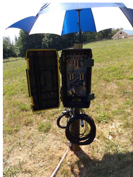
Box under antennas, with the "Service shelter"
