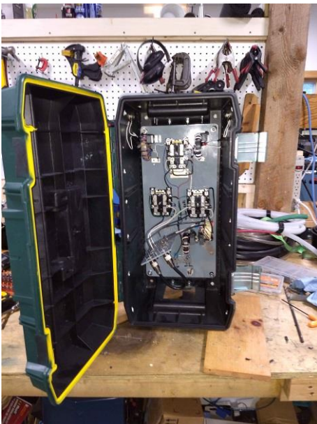
Inside control box
